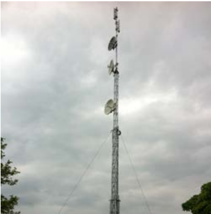
Rocket M5 access points attached to RocketDishes and sector antennas
